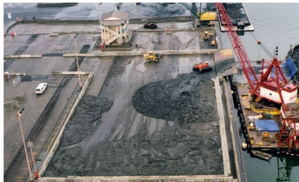
Contained landside facility
